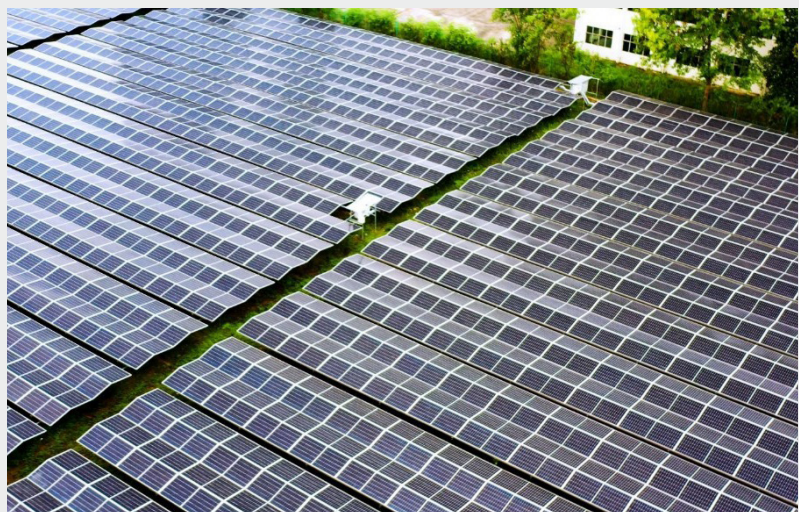
Solar panel installation at Benoi under the SolarLand programme
